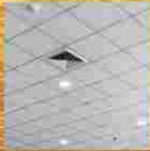
CEILING GRID FALSE CEILING
