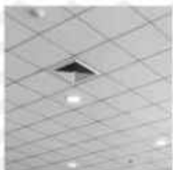
CEILING GRID FALSE CEILING
