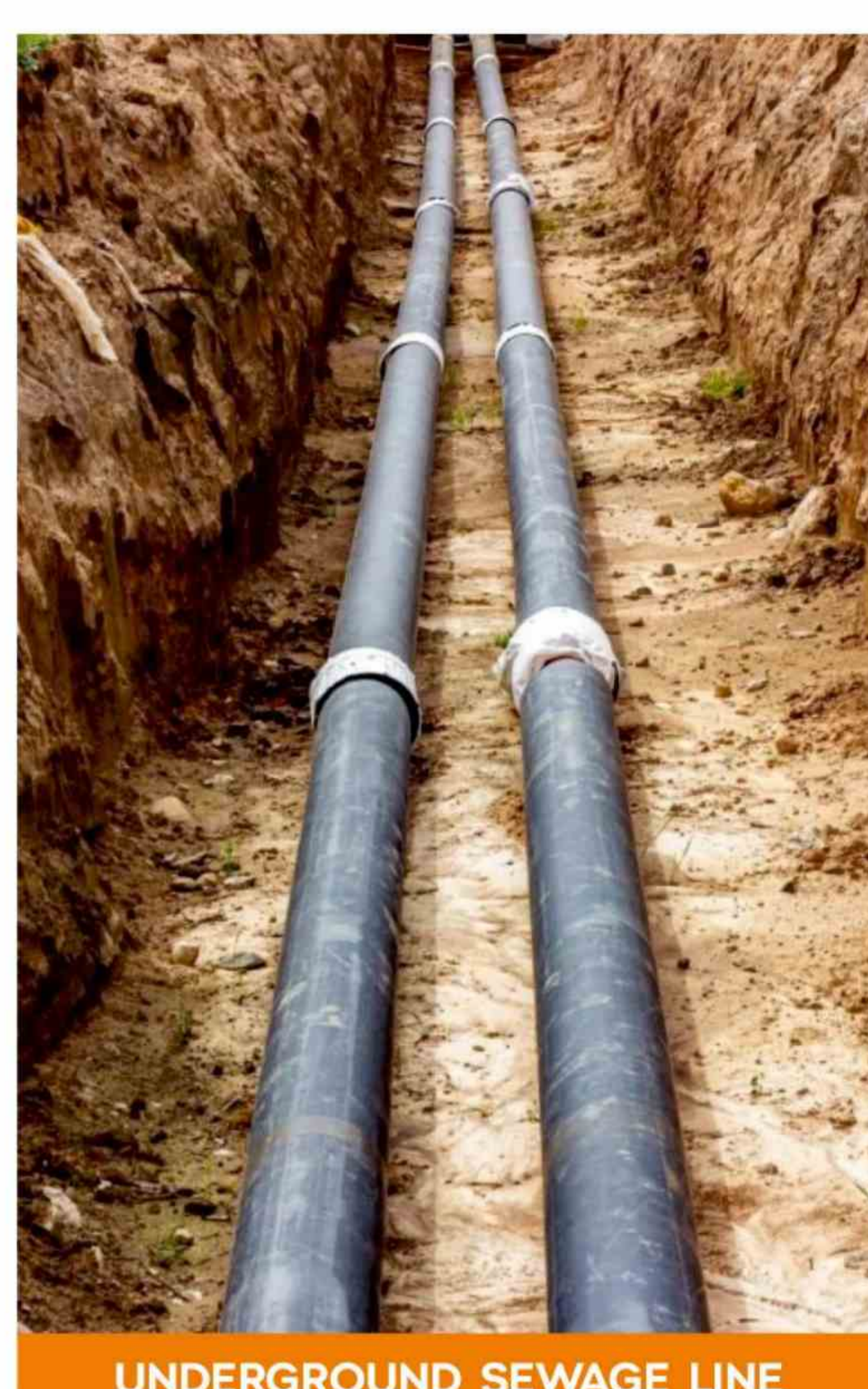
UNDERGROUND SEWAGE LINE
