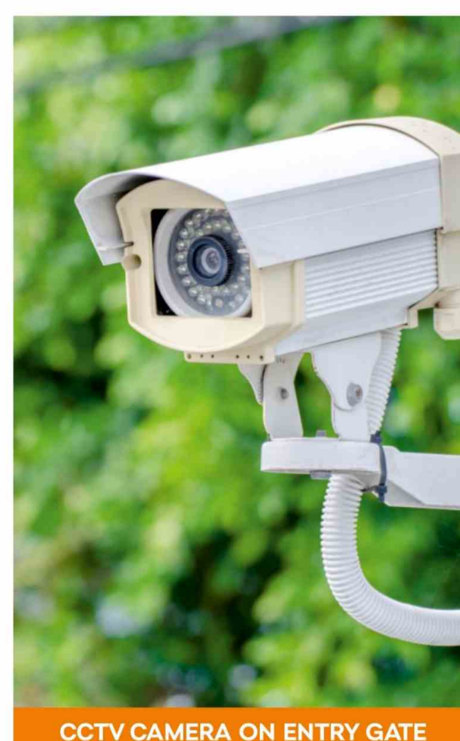
CCTV CAMERA ON ENTRY GATE
