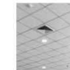
CEILING GRID FALSE CEILING
