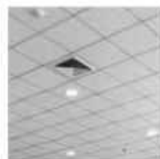
CEILING GRID FALSE CEILING
