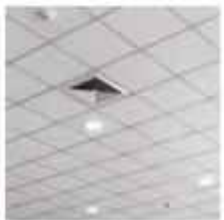
CEILING GRID FALSE CEILING
